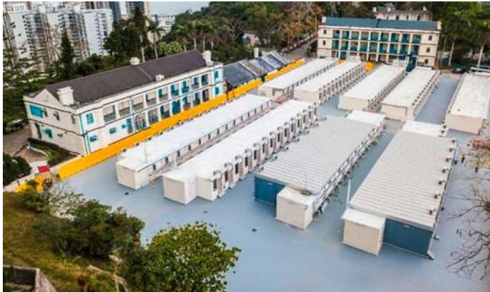
Figure 25. Upper Lei Yue Mun Park – Basketball Court, with 118 units in single storey high, completed in February 2020 in 26 days.
