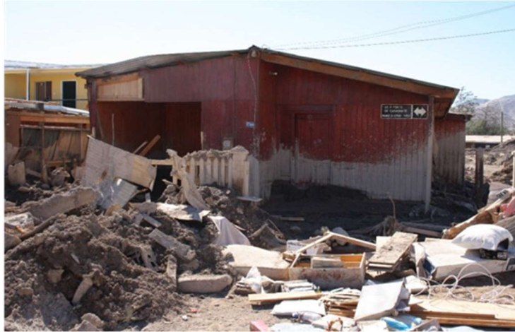
Figure 15. House obstructed by debris left by the alluvium, Copiapó, March 2015 (Photo: C. Jiménez)
