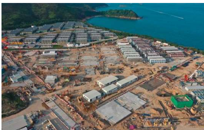
Figure 31. Penny's Bay Phases 3 and 4, with 2000 units in 2 storeys high, are under construction, and target to be completed in the end of this year.
